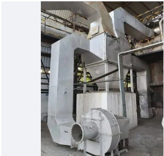
Air Preheater for Boilers
