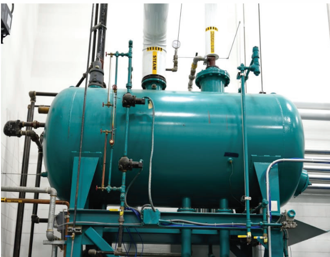
Feed Water Tanks
